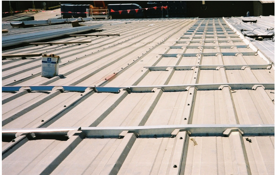
JG Smith Construction tried different methods of installation, but found the Roof Hugger to be the most efficient metal roofing retrofit system for its uses at the Mills Pride furniture manufacturing complex in Waverly, Ohio. JG SMITH CONSTRUCTION PHOTOS
