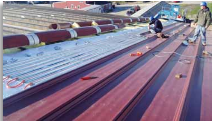
Actual construction of a "SWH" system over a metal roof with fiberglass insulation between the existing metal roof and bottom of solar tubing. New roof panels are being installed.
