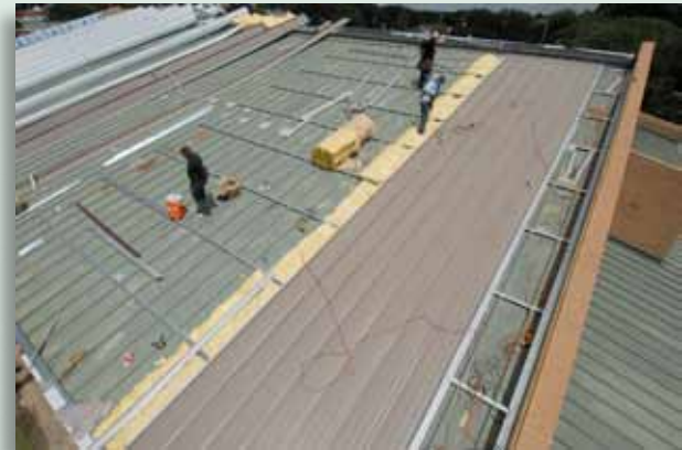
New metal roof and Roof Hugger sub-purlins installed over existing metal roof and "ASV" air-space above new fiberglass insulation.
