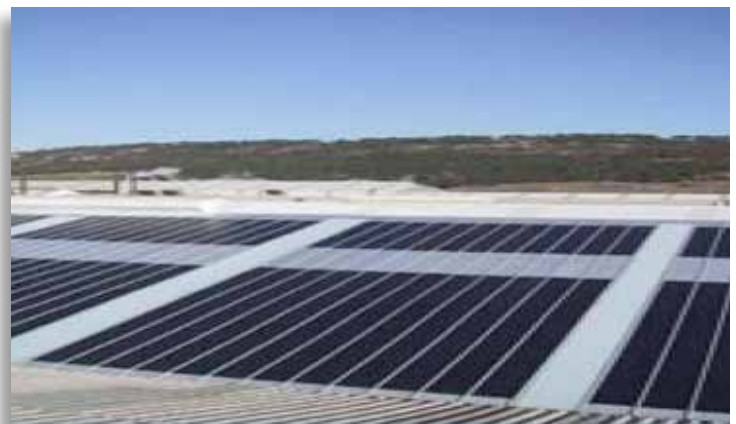
A Solar Photovoltaic (PV) energy system installed over a metal roof.
